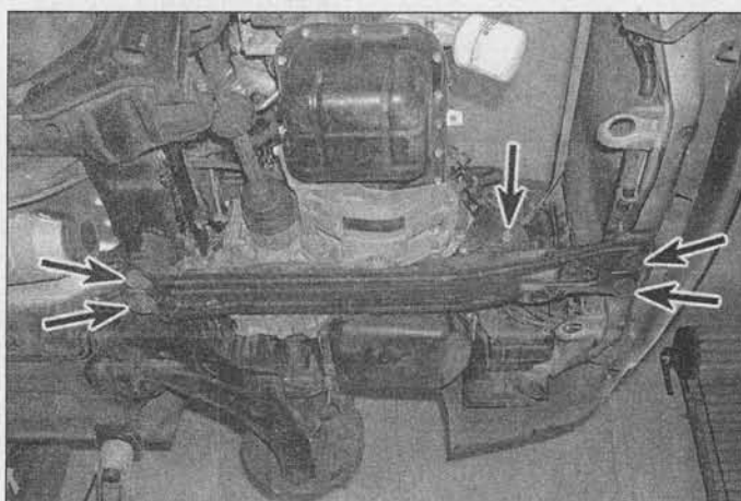
6.11 On 2000 and earlier models, remove the bolts from the transaxle roll stopper and the center member (arrows)
